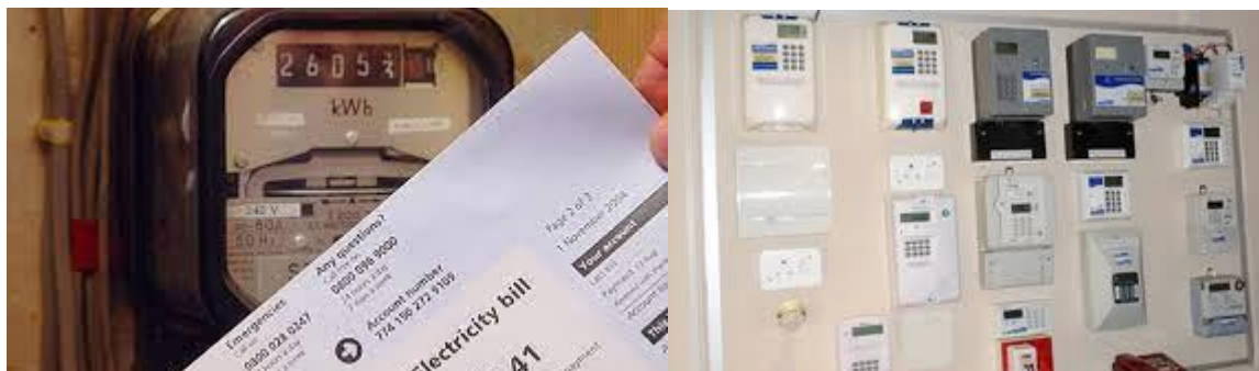
Figure 4: Estimated electricity billing devices – Post Paid
